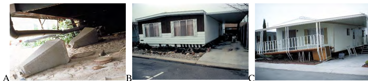
Figure 2-54: Earthquake damage to manufactured housing. (A): Overturned concrete piers that supported a manufactured house, viewed after the 1978 Santa Barbara earthquake. (B) and (C): Collapsed manufactured houses after the 1980 Livermore earthquake. (Images courtesy of National Information Service for Earthquake Engineering, University of California, Berkeley.)
