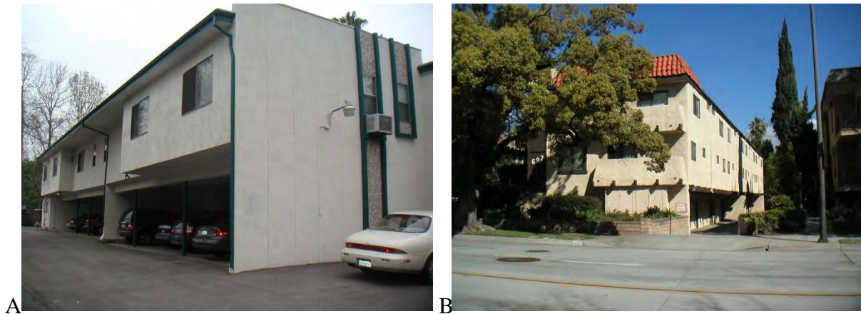
Figure 2-49: Soft-story wood-frame multifamily dwellings. (A) Menlo Park, California. (B) Pasadena, California. (Photo credit: Porter 2006, used with permission.)
