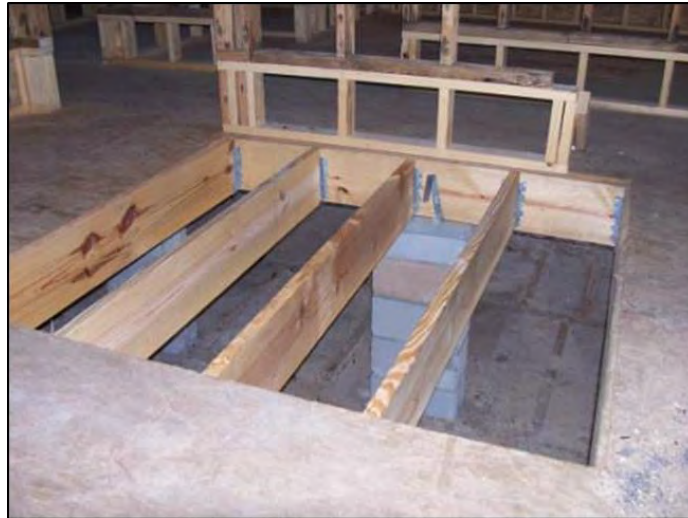
Figure 2-35: Examples of elevated single-family house where the walls were separated from the slab and a new wood-framed floor system was constructed (Source: John Squerciati)
