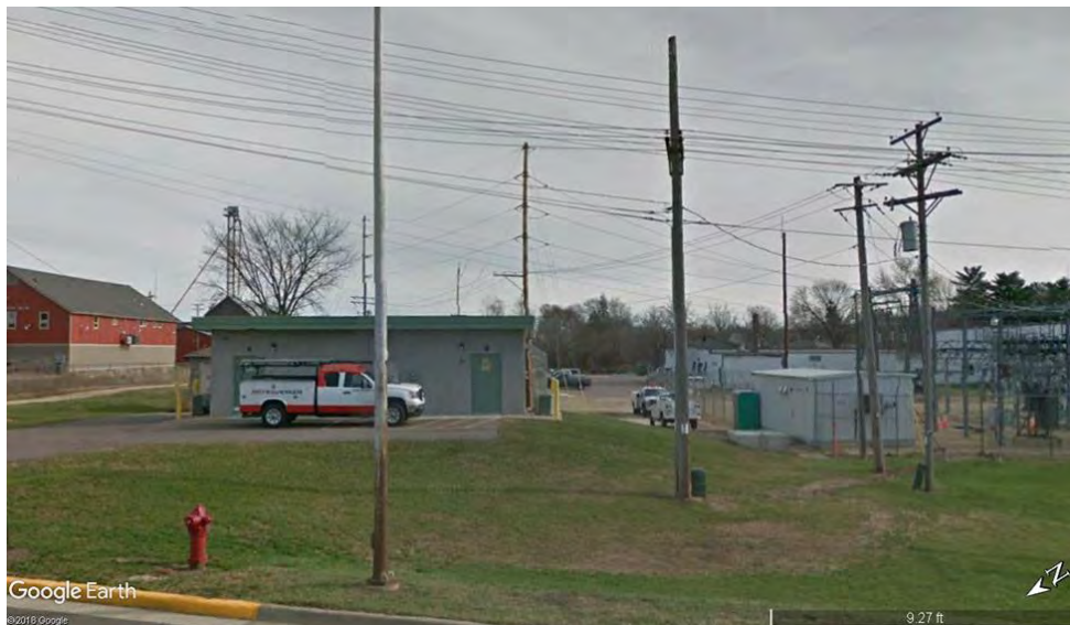
Figure 6-21: Electrical and telephone switching stations in Reedsburg, Wisconsin. The old one is to the right with the green cabinet next to it; the new one is to the left, behind the pickup truck.
