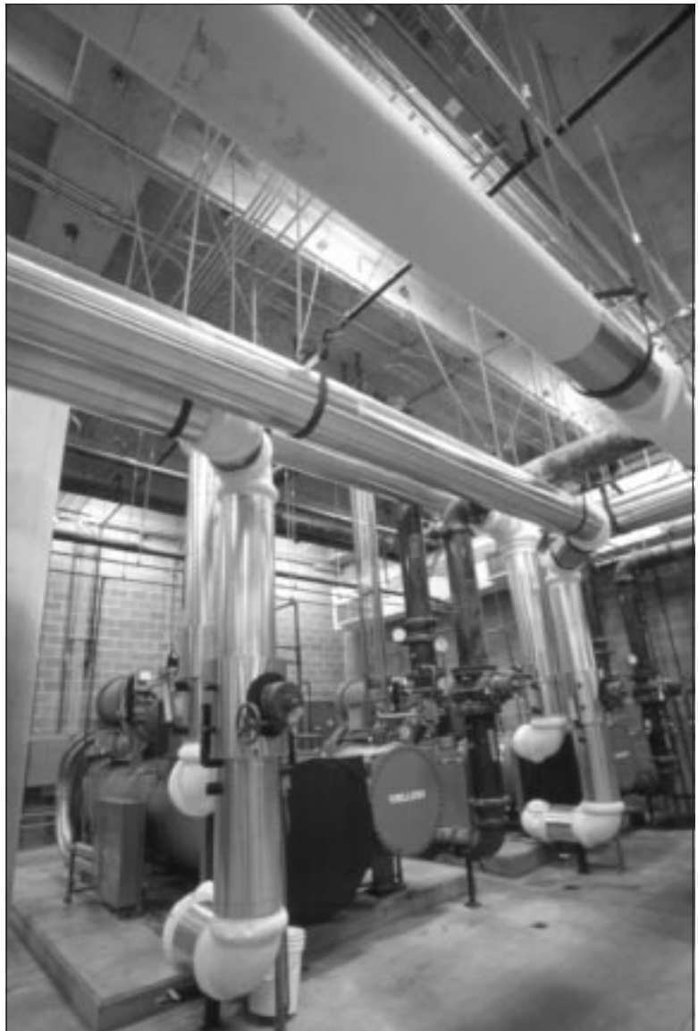
The immaculate chiller room at DLA is adjacent to the underground ice plant
