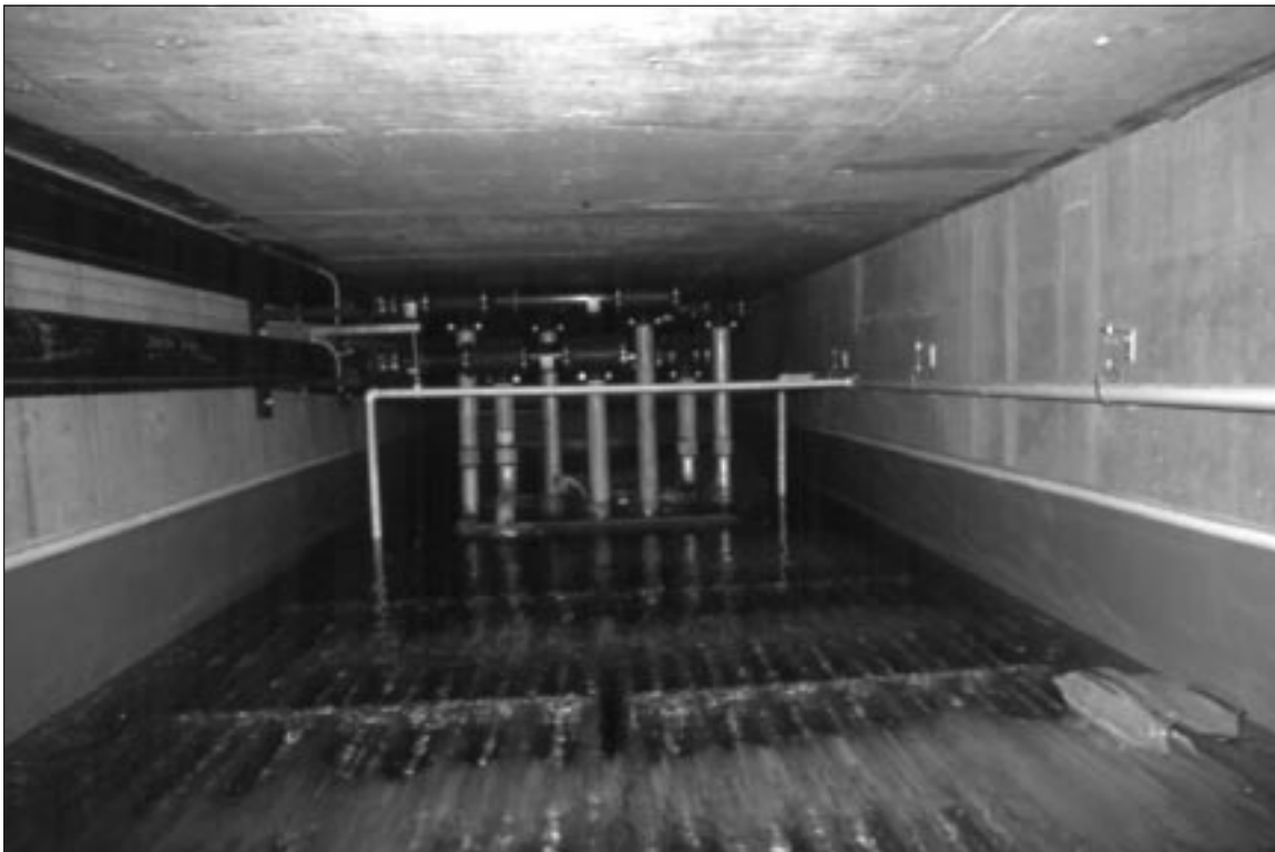
This “ice plant” is the heart of energy conservation for the DLA building. It has the capacity to provide “primary” cooling for substantial periods.
