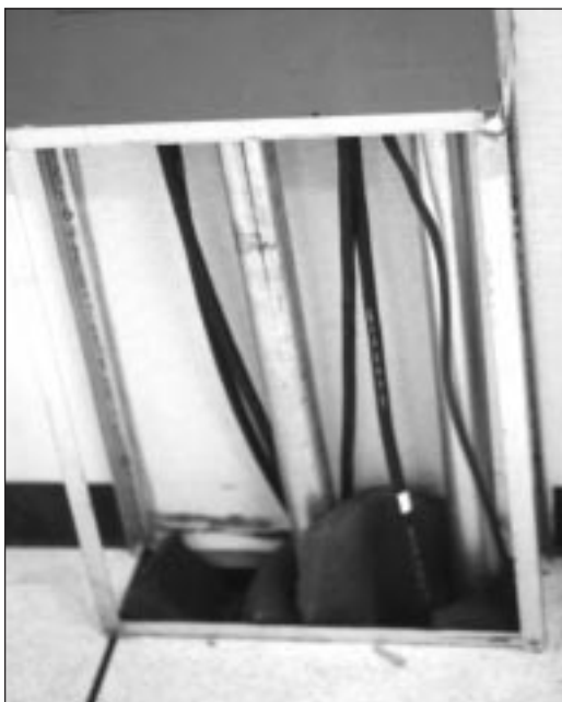
This simple method of insulating cabinets resulted in both cooling and heating savings.
