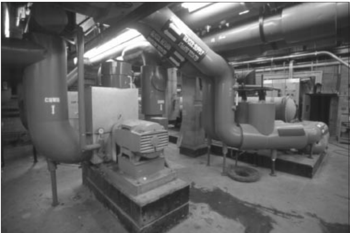
All USDA mechanical rooms were cleaned and polished as part of the maintenance upgrade. This spotless new chiller for the ice plant reflects the current conditions.
