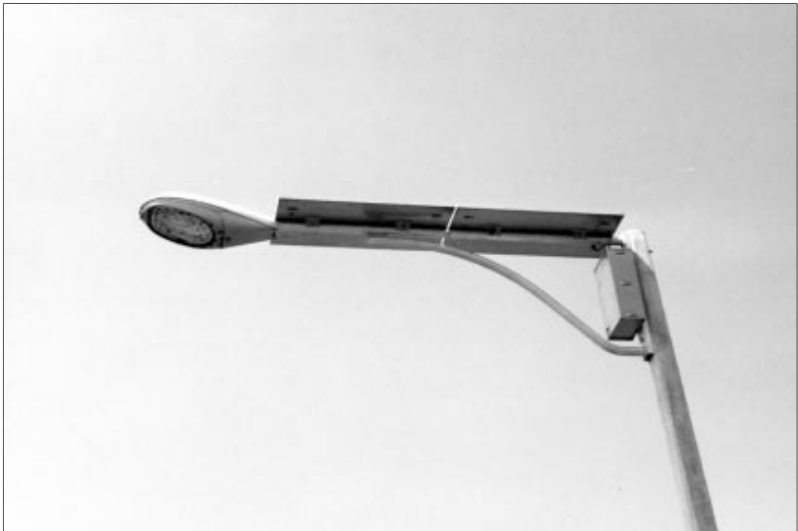
Photo-voltaic panels provide solar power for perimeter lights.
