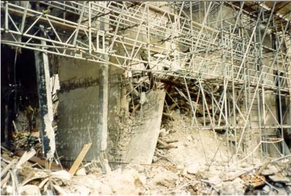
Figure 4. Damage to ground floor columns –Kansallis House, Bishopsgate
