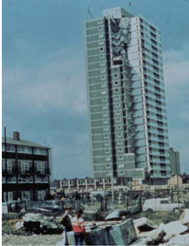
Figure 1. Progressive collapse - Ronan Point.
