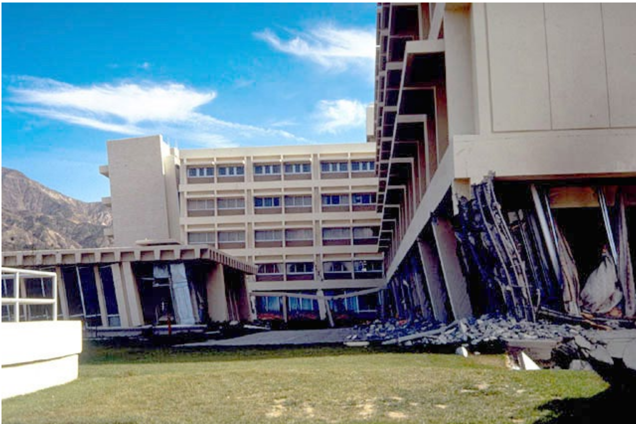
Figure 3-11. The extreme drift or sideways distortion of the Olive View Hospital in the 1971 San Fernando was caused by a soft-story condition: strong and stiff walls were discontinued at the ground story level, and all of the deformation was imposed on the columns. (Source: William Godden, NISEE-PEER )
