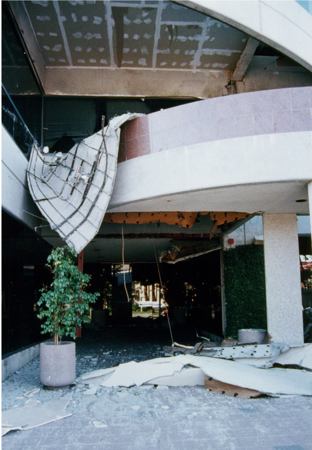
Figure 3-10. In the 1994 Northridge Earthquake in the Los Angeles region, this heavy soffit or exterior ceiling collapsed over the entrance. Nonstructural protection involves secure attachments of the nonstructural components to the structure. (Source: Robert Reitherman)
