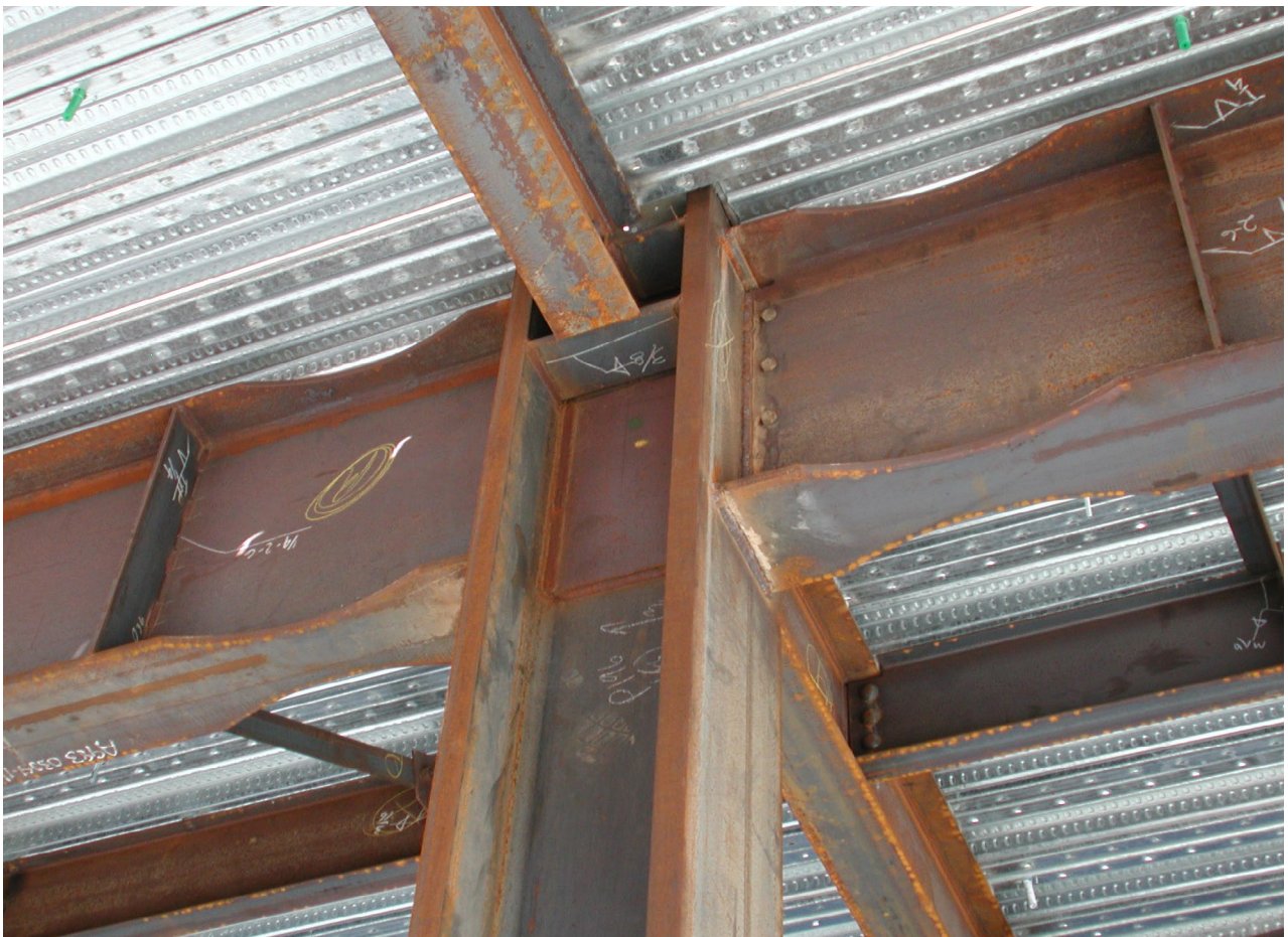
Figure 3-5. In this technique for allowing a steel frame to deform in a ductile manner, the beam is intentionally weakened with a “dogbone” cutout so that inelastic behavior will be concentrated in that segment of the frame, protecting the column from damage. (Source: Chia-Ming Uang)
