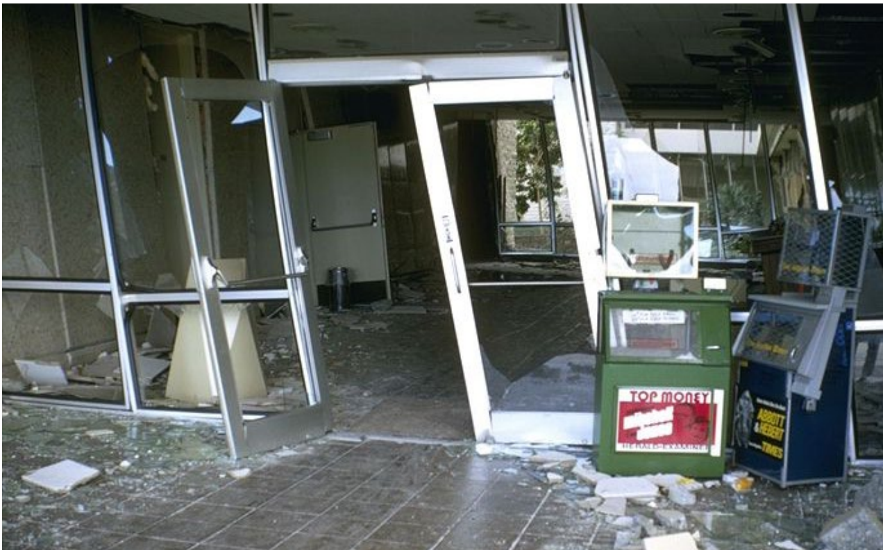
Figure 3-9. The extreme drift and structural damage experienced by Olive View Hospital in the 1971 San Fernando Earthquake also rendered nonstructural components damaged and non-functional. (Source: Robert Olson, NISEE-PEER )
