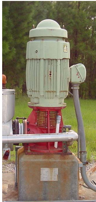
Figure 4.1-14 Vertical Sump Pump Motor
