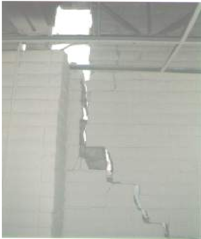
Figure 9.1-2 Seismic Induced Failure of Block Walls
