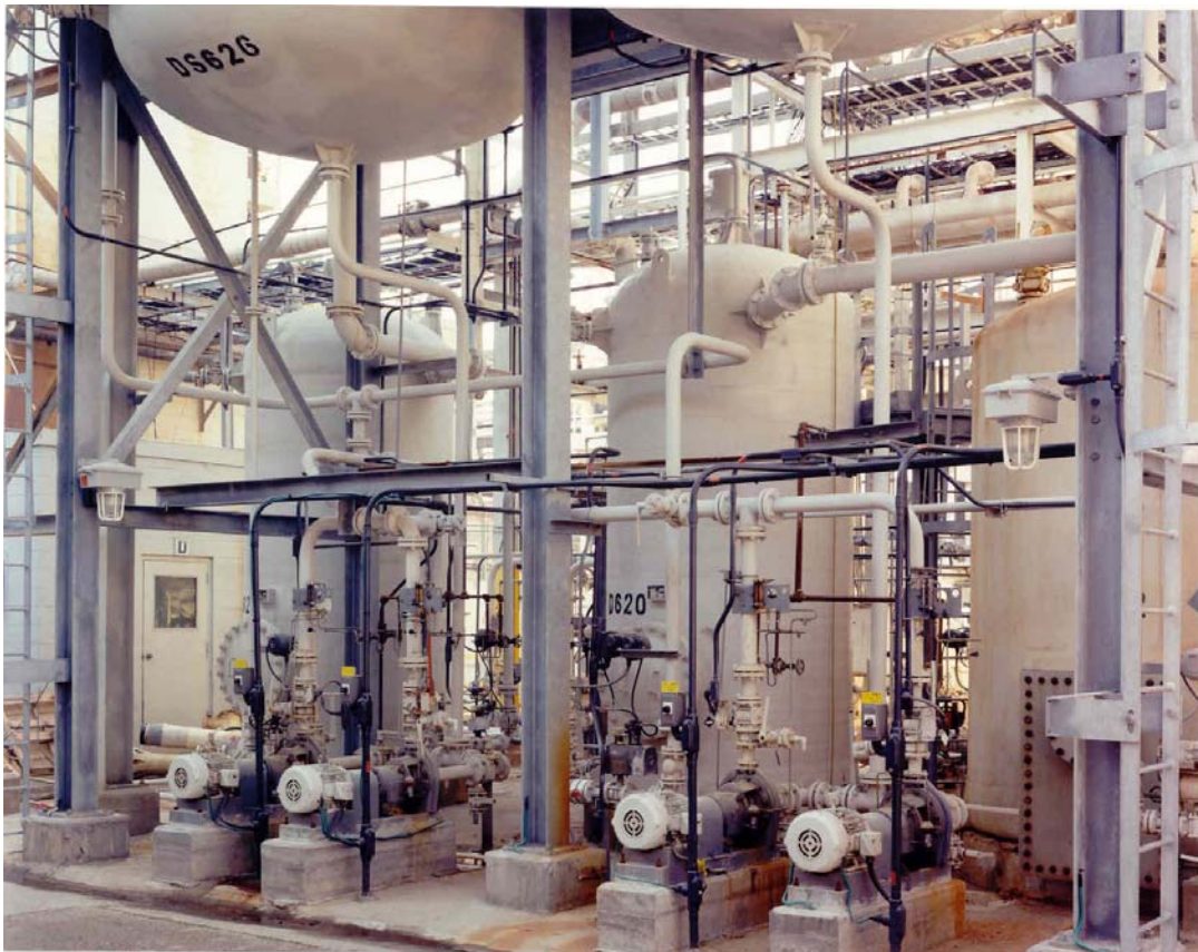
Figure 4.1-11 Four Centrifugal Horizontal Pumps on Concrete Pedestals
