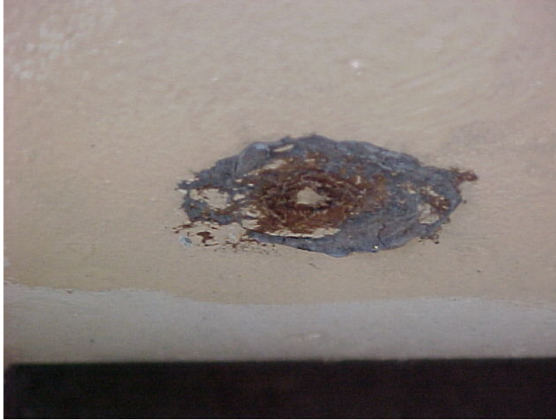
Figure 5.5-2 Corrosion in Air Receiver Tank of Outdoor Air Compressor Unit
