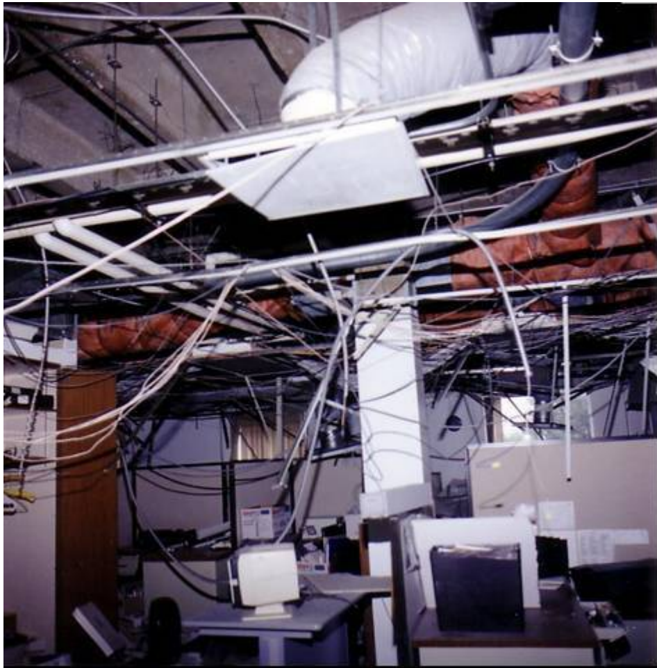
Figure 9.7-2 Fall of Overhead Suspended Ceiling
