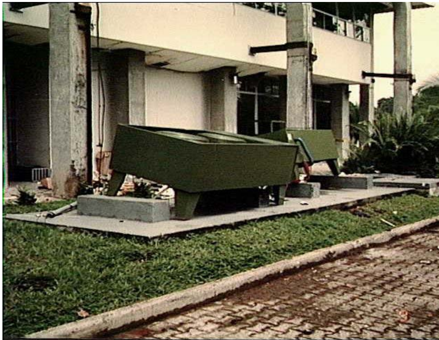
Figure 6.2-9 Unit Slides off Pedestal
