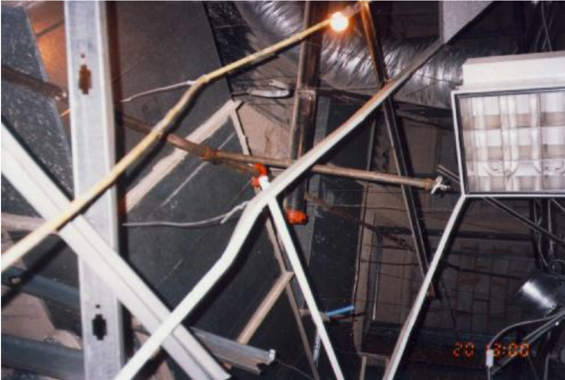
Figure 9.1-1 Seismic Induced Failure of Suspended Ceiling
