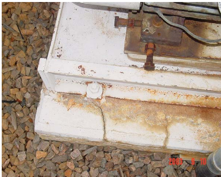
Figure 8.6-1 Crack in Concrete Pad Through Bolt
