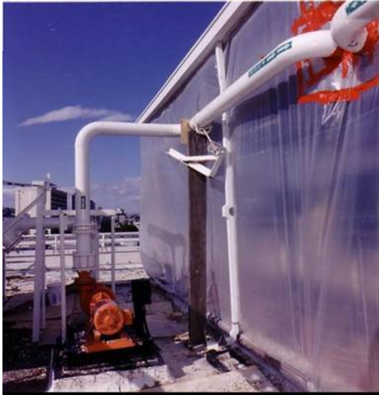
Figure 4.2-4 Failed Pipe Support on Pump Discharge
