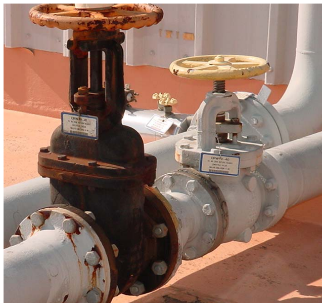
Figure 3.5-2 External Corrosion Unpainted Valve
