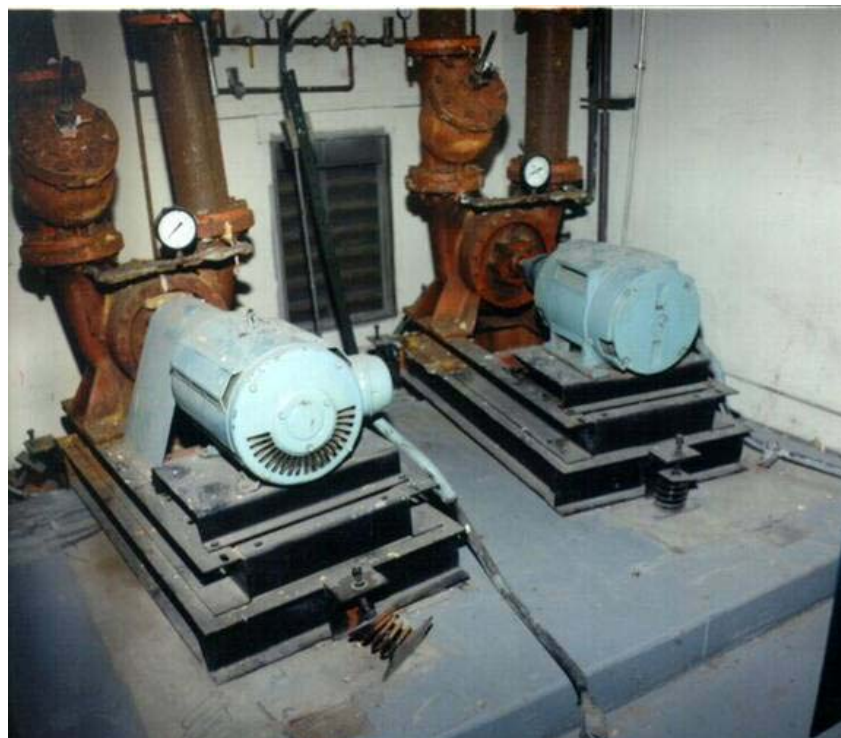
Figure 4.2-7 Vibration Isolator Failure at Left
