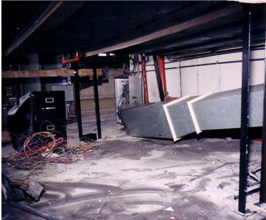
Figure 6.2-10 Falling of Overhead Duct (Mason Industries)
