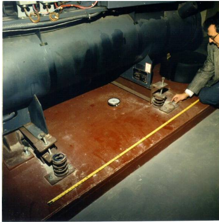
Figure 7.2-1 Failed Vibration Isolators (Mason Industries)
