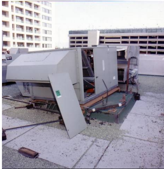
Figure 6.2-6 Damage Caused by Failure of Spring Mounts (Mason Industries)
