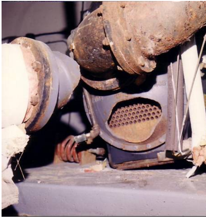
Figure 4.2-12 Tearing Rupture of Heat Exchanger Nozzle (Mason Industries)
