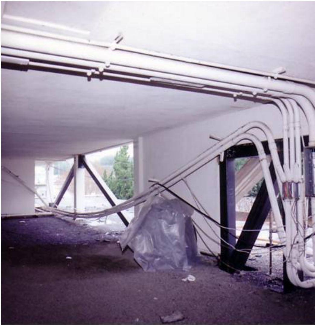
Figure 9.7-1 Fall of Overhead Pipe or Conduit
