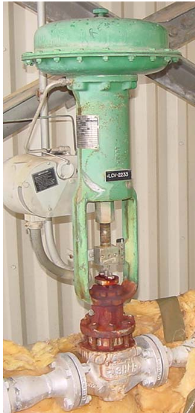
Figure 3.4-1 Air Operated Valve with Eccentric Operator
