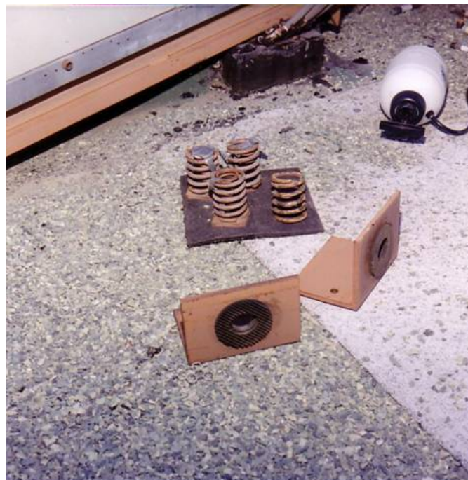
Figure 6.2-7 Failure of Spring Isolators (Mason Industries)
