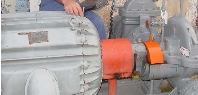
Figure 4.5-1 Horizontal Pump Vibration Reading
