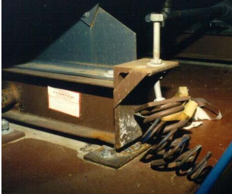
Figure 8.3-2 Failed Spring Vibration Isolator (Mason Industries)
