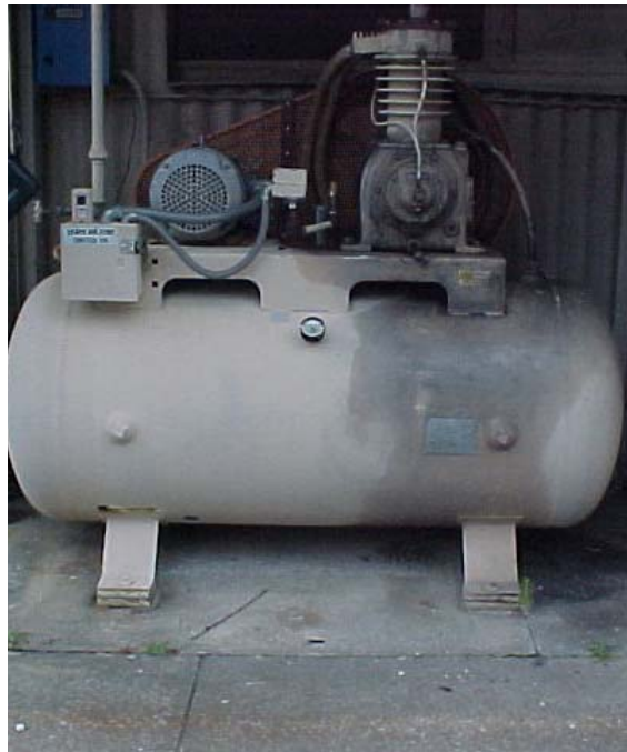
Figure 5.5-1 Reciprocating Compressor atop Air Receiver
