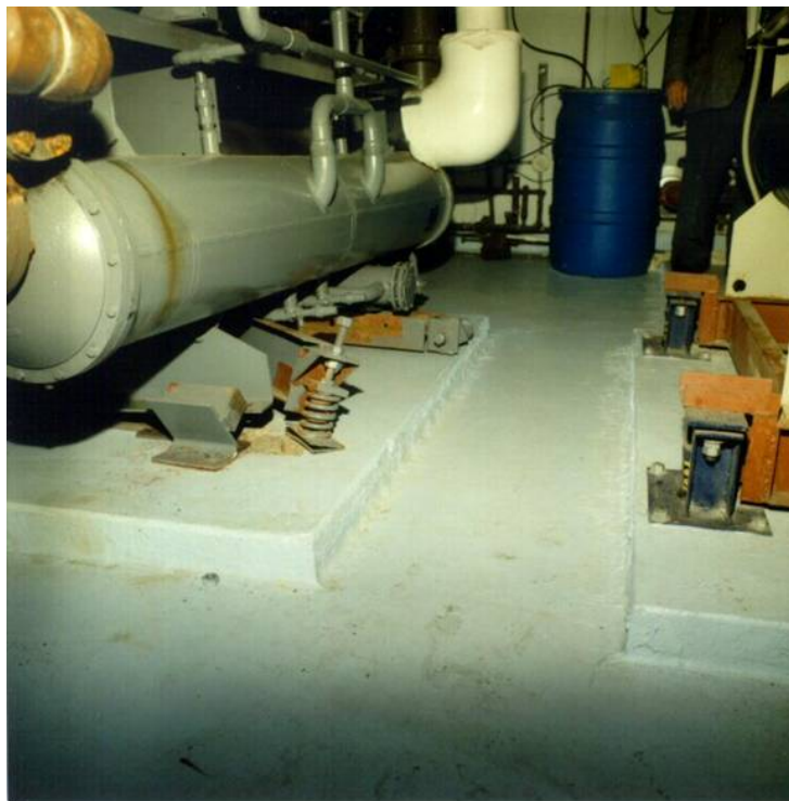
Figure 7.2-2 Failed Vibration Isolators (Mason Industries)
