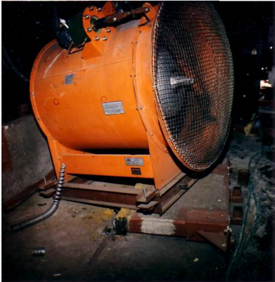
Figure 6.2-5 Failure of Spring Mounts (Mason Industries)
