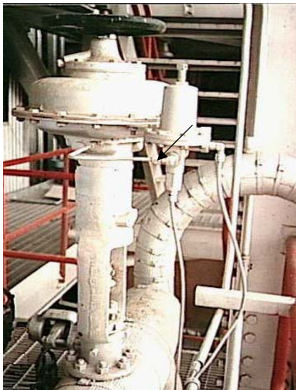
Figure 3.2-4 Failed Air Supply Tubing After Repair (ABS Consulting)
