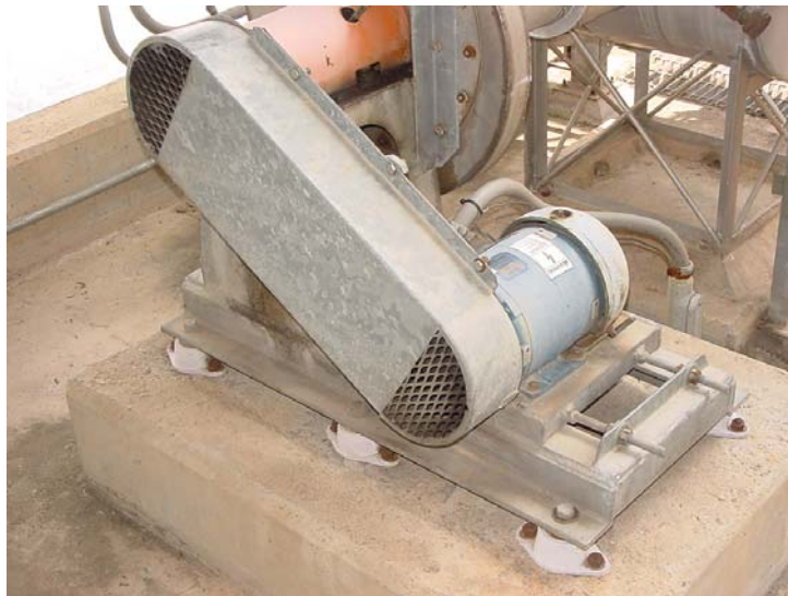
Figure 6.1-4 Fan on Vibration Isolation Springs
