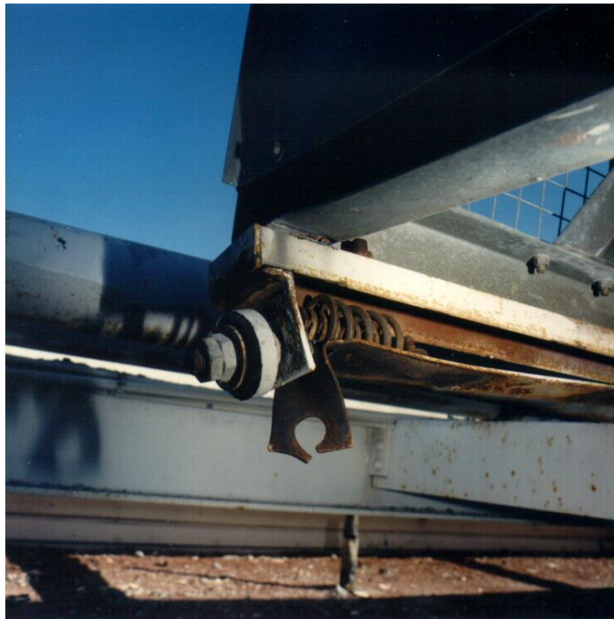
Figure 6.2-4 Failure of Spring Isolator (Mason Industries)
