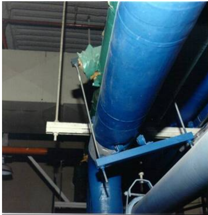
Figure 4.2-3 Pipe Support Failure (Mason Industries)
