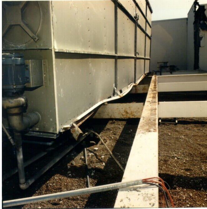
Figure 6.2-3 Shift of Roof-Top Unit (Mason Industries)
