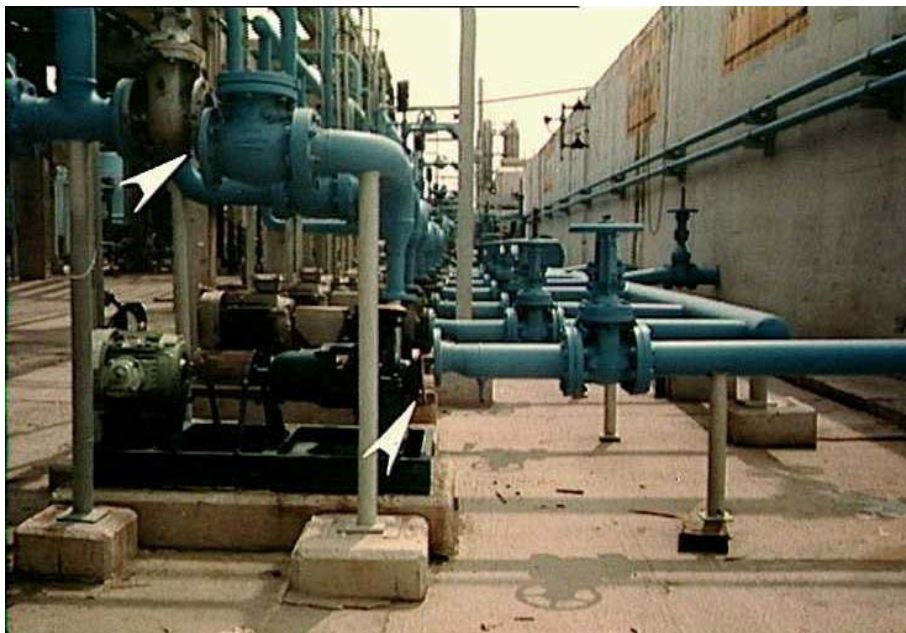
Figure 4.2-1 Seismic Ground Settlement (ABS Consulting)
