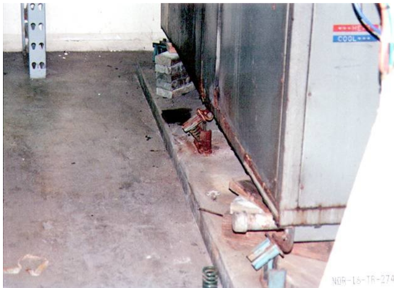
Figure 6.2-2 Failure of spring isolators (ABS Consulting)
