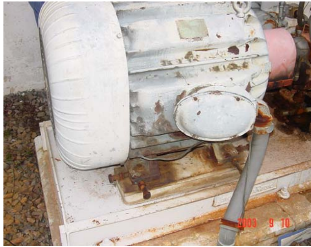
Figure 4.5-3 Corroded Pump Base and Alignment Pins
